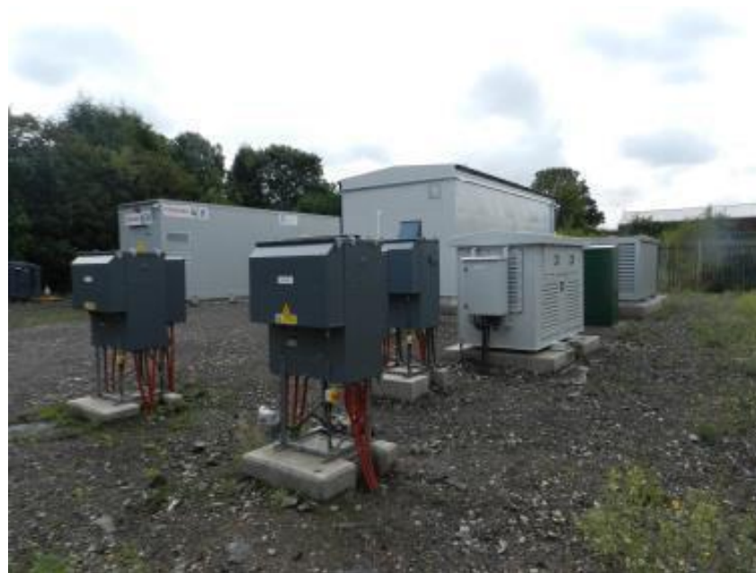
Willenhall Battery 2MW, 1MWh Toshiba lithium titanate battery system
